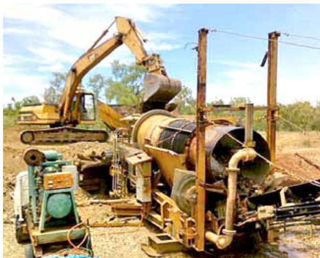
ERO gold trommel wash plant showing alluvial gravels from excavator to conveyors, November 2010.
